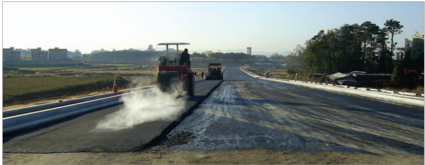
Work under way for a road leading to the newly built U.S. military base in Pyeongtaek (Camp Humphreys, December 2008)
